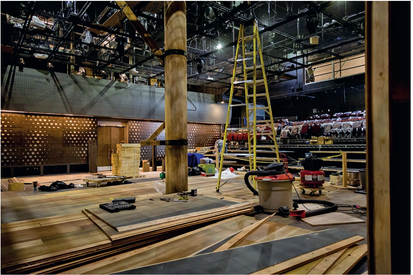
Construction on the Goldcorp Stage at the BMO Theatre Centre in South False Creek. Photo by Mark Halliday
