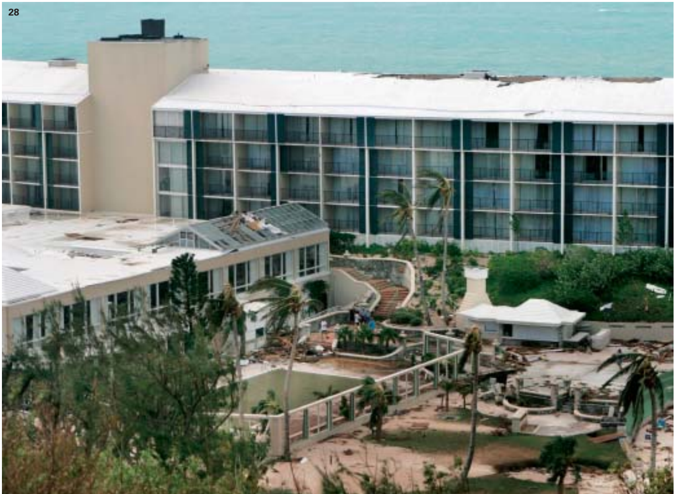
Wind and storm surge damage at a hotel complex in the Bermudas. The damage caused by Hurricane Fabian reached from the roof of this complex to its foundations.
