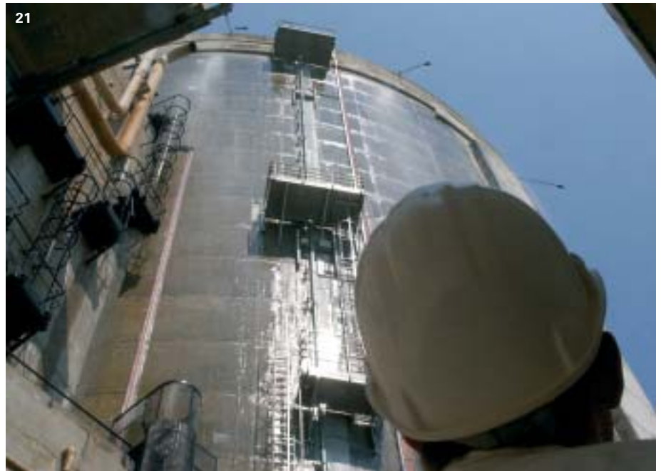
At the peak of the heat wave, water had to be sprayed onto the outside surfaces of numerous power plants above ground (as here in Fessenheim, France) as the cooling systems were no longer working efficiently due to the heated rivers and the shortage of water. Some power plants had to reduce their output, some had to be shut down altogether.
