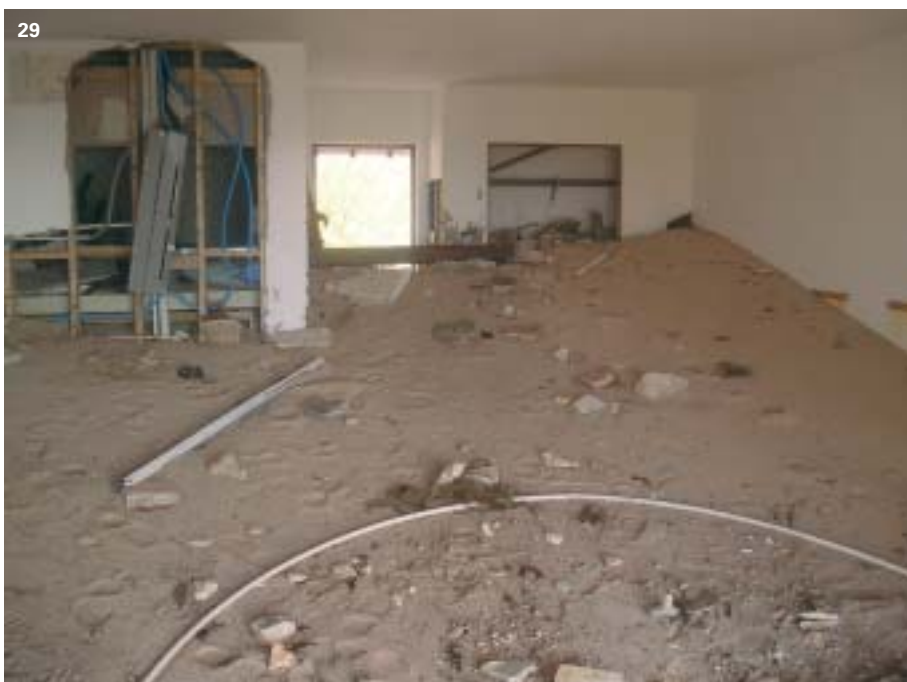
The storm surge whipped up by Hurricane Fabian washed sand and rubble into numerous buildings near the shore. Even if high wind-load standards are incorporated in the building code, they will not reduce such losses to any substantial degree.
