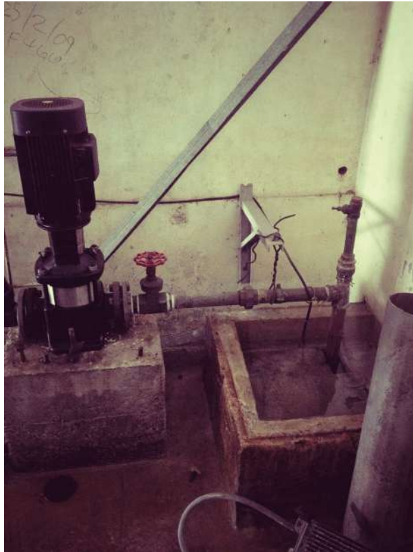
Figure 3: Motorized water pump at ground level in my residence
