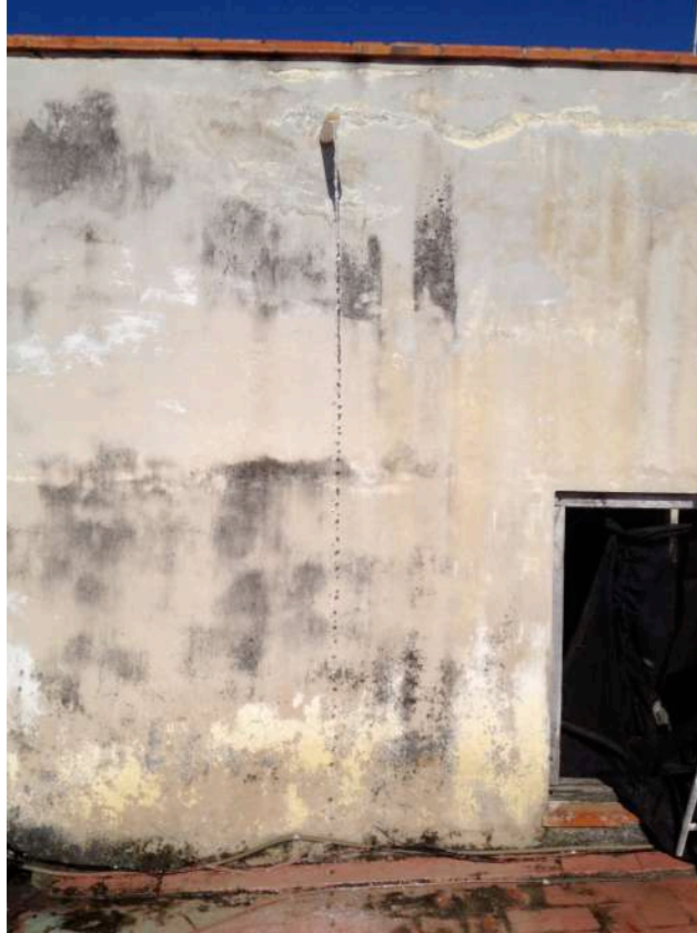
Figure 4: Water overflowing from the spout of the rooftop reservoir
